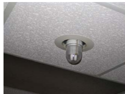
A Dress up ring from Home Depot and the 12 volt light on the left makes a perfect installation
